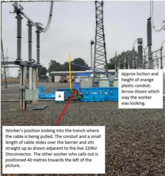
Figure 1 - Yellow markup is simulating the conduit snake proximity to 220kv disconnector
