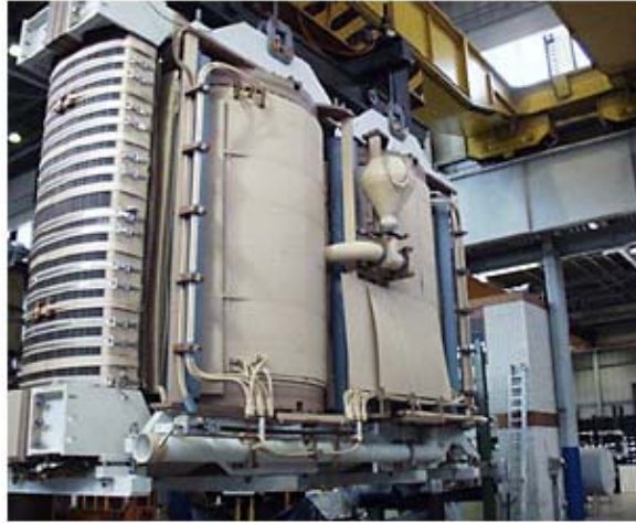
Courtesy Smit Transformers
