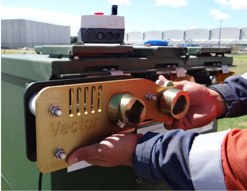
Figure 8 Portable Actuator ready to operate the Earth switch
