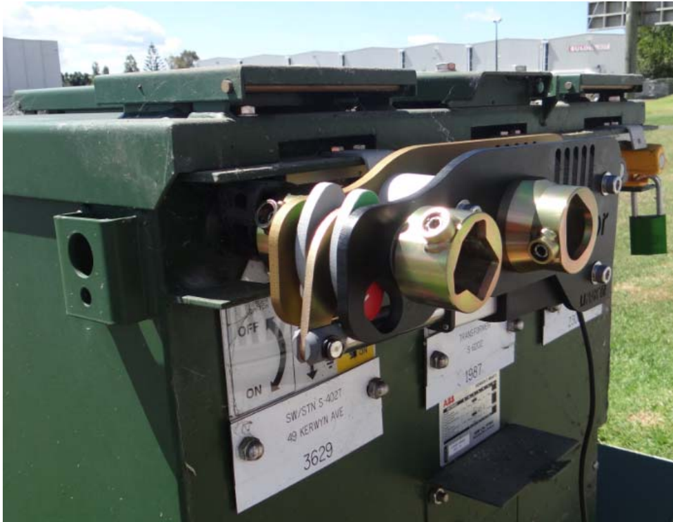
Figure 6 Portable Actuator ready to operate the Isolator switch
