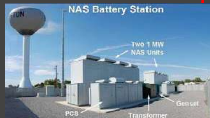
Substation Batteries 10s of MW
