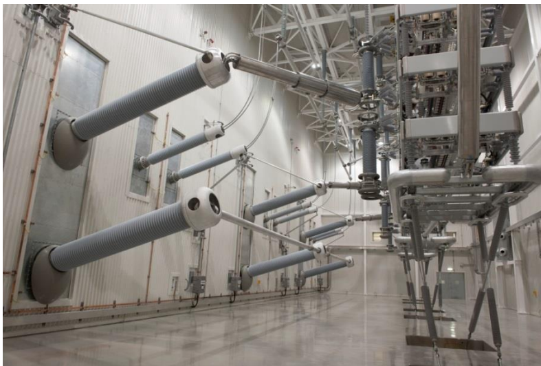
Figure 2: Converter transformer bushings
