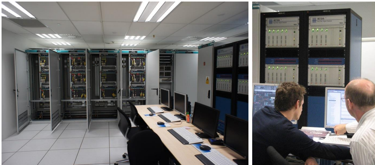
Figure 5: Transpower's GHOST (Grid HVDC Offline Simulator Tool) installed in Wellington
