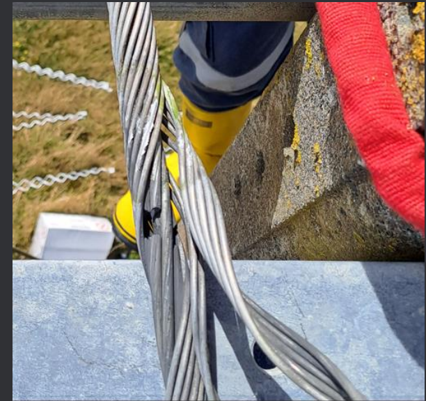
Aeolian vibration damage
