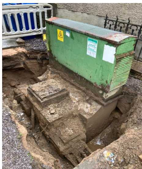
Example unit with enclosed pipework
