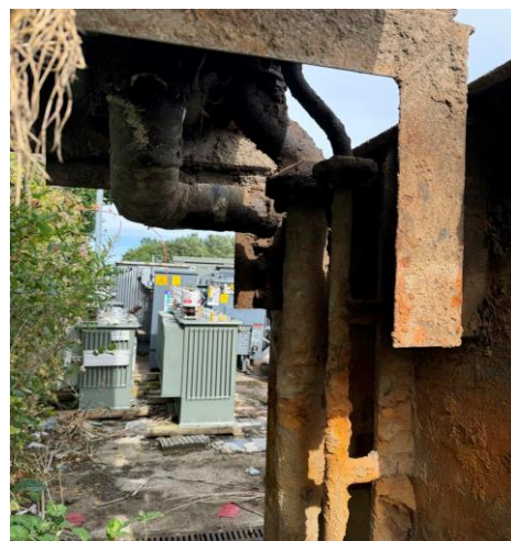
Example unit with exposed pipework
