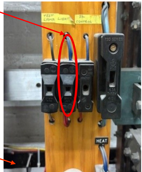
Photo A Battery charger isolation fuse (centre) labelled 'Light'
