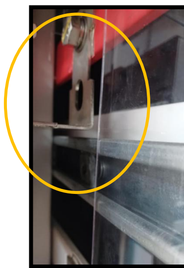
Potential arc flashpoint
