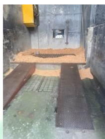
Fuel unloading bunker at DEC — grate and unloading zone.
