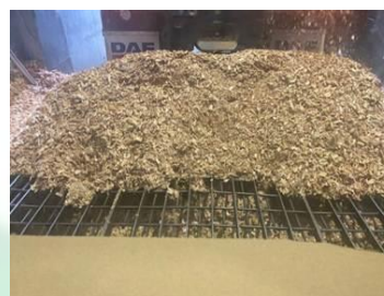
Woodchip bridging on the grate above the fuel hopper.
