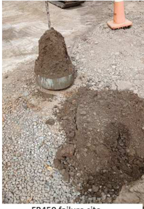
FB450 failure site
