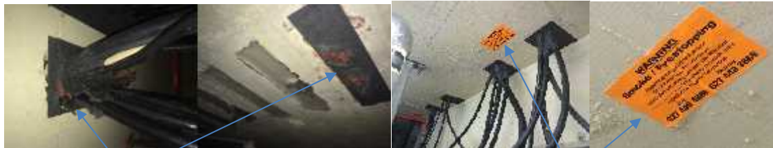
Fire Seal damage alongside a compliant seal and warning notice label
