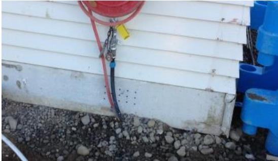
Asbestos baseboards, soffits, cladding etc
