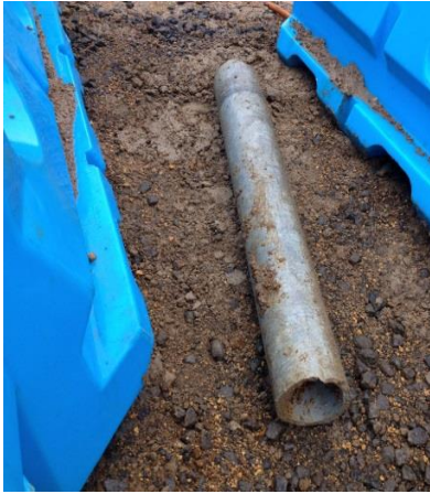
Water pipes, storm water, gutters, down pipes
