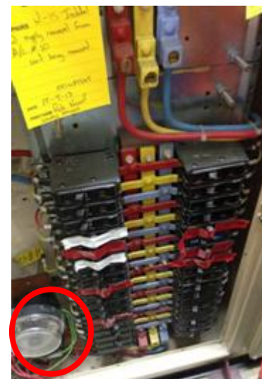
Breakers located in DB31 Position of Live cables circled
