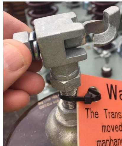
Figure 3: Broken Eyebolt on MV Bushing
