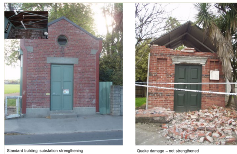
Figure 25: Substation Damage Comparison
