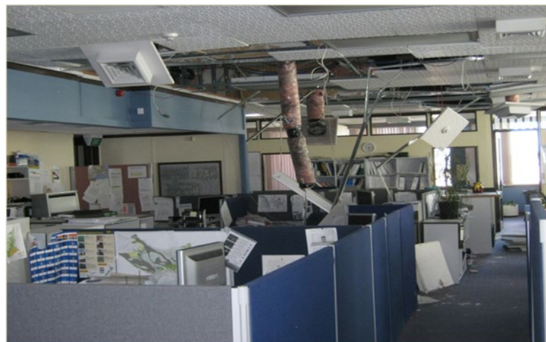
Figure: 29: Second Floor Office Damage
