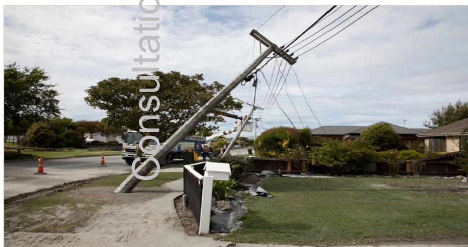
Figure 22: Low Voltage Line Damage
