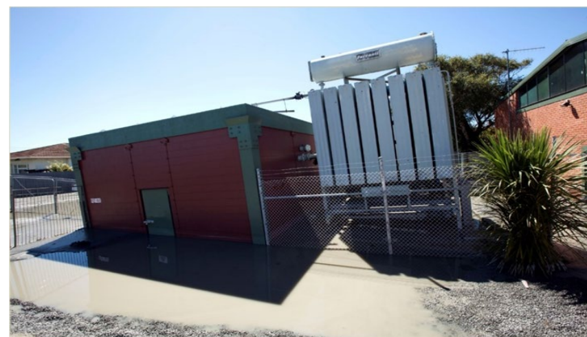
Figure 23: Liquefaction Impact on Major Substation
