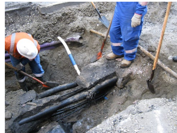
Figure 21: 66kV Cable Damage
