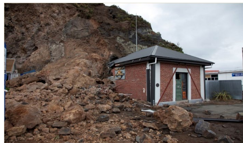
Figure 27: Substation Rock Fall Damage
