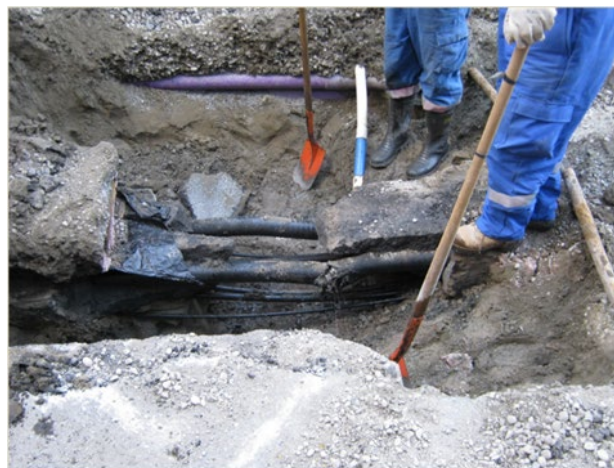
Figure 20: 66kV Oil Filled Cable Damage – Armagh Street
