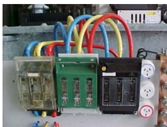
A set of 3 horizontal disconnects. The Jean Muller unit is the one on the right hand side. The locking mechanism is on the top left hand corner. It is in the unlocked position. There is no lock on the other two disconnects.
