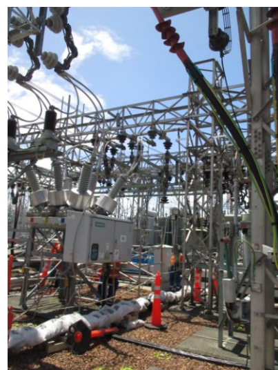
Photo of circuit, note that the position of the staff member is where the operator would be
