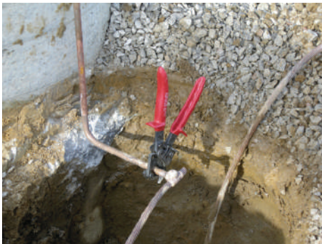
Unsuccessful attempt to steal copper within a substation
