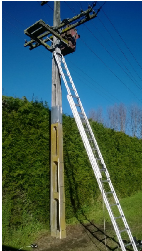
Photo 1: The accident scene.
